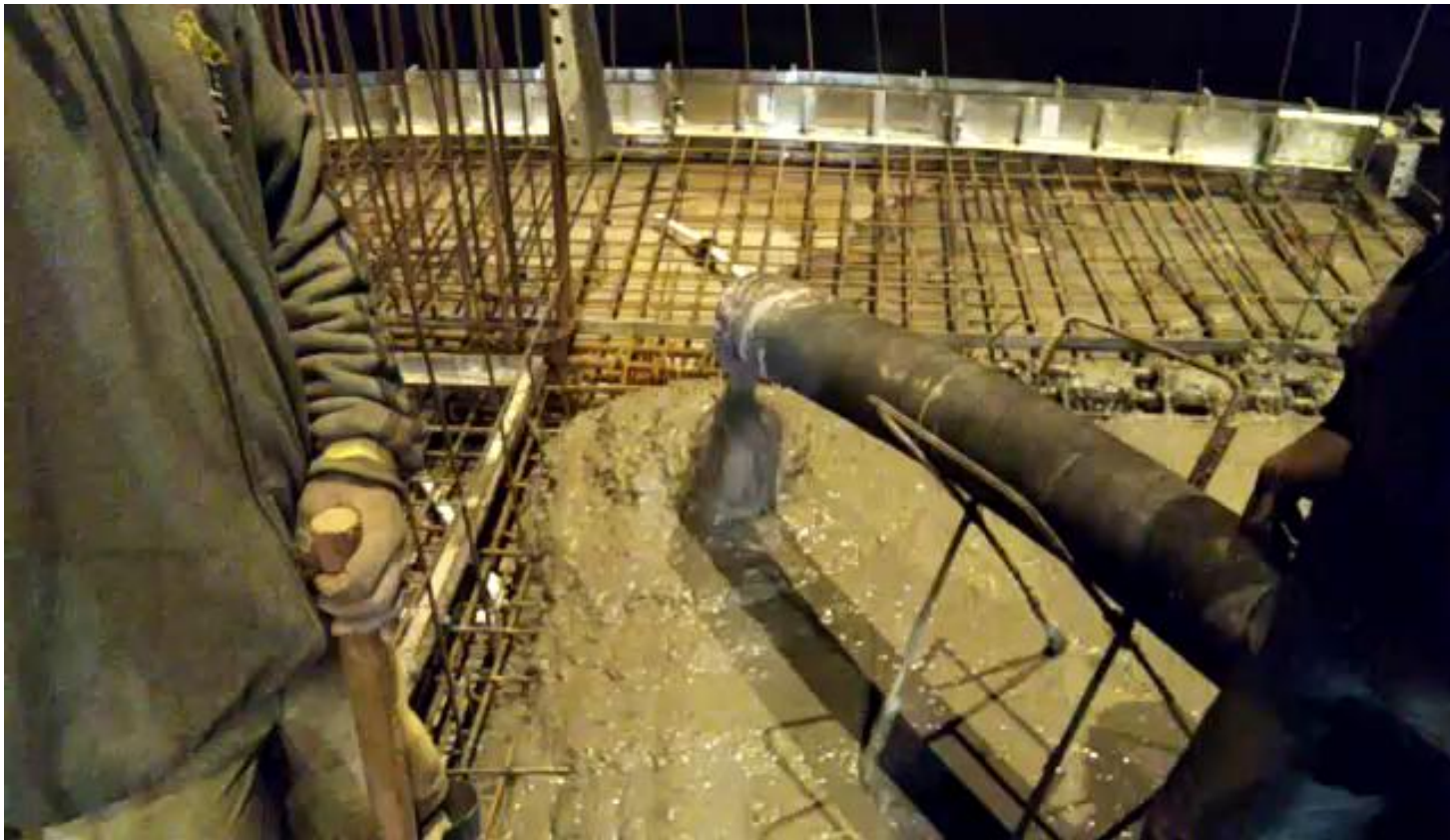
Wrong Placing of Concrete
