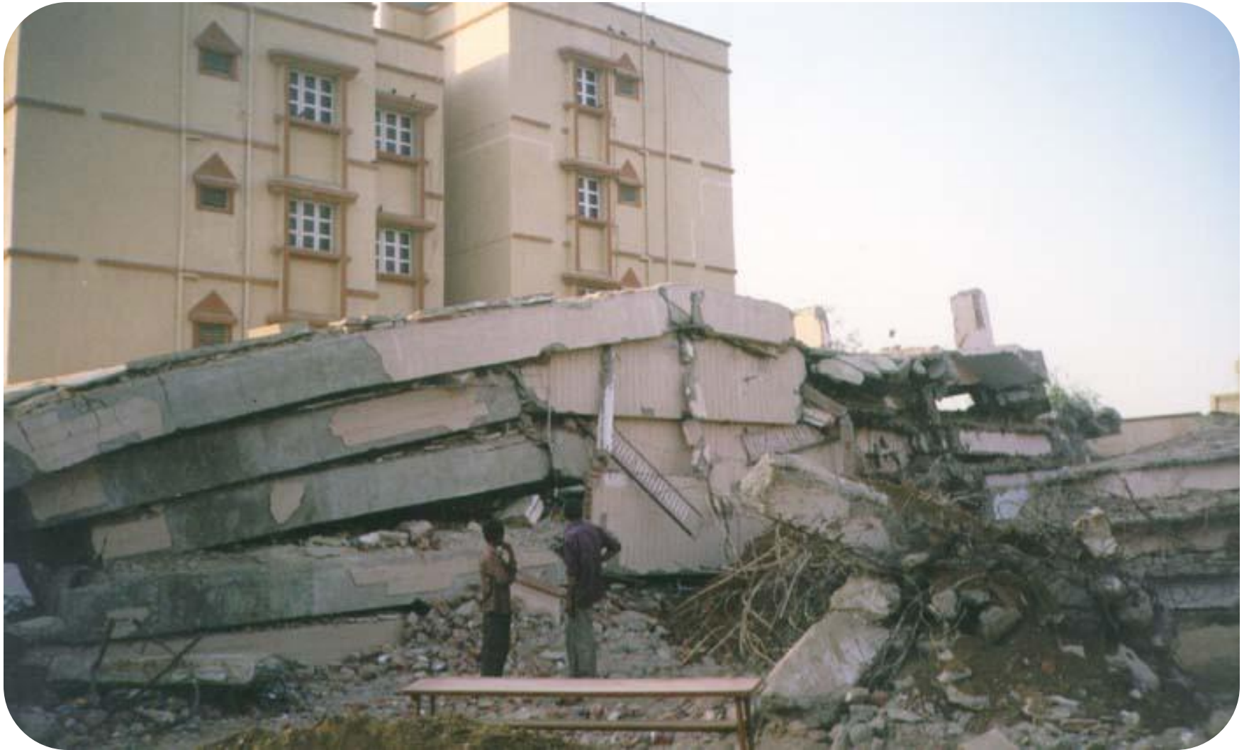
Figure: Damage to Ground Floor Columns Due to Inadequate Lateral Confinement of Reinforcement bar
